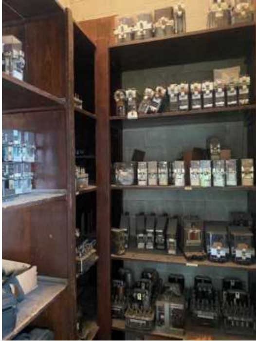
This closet on the second floor was full of electrical switches, relays and other electrical components. Another closet on the second floor held multiple large industrial batteries for backup to the physical plant and signals in case of a power failure.
