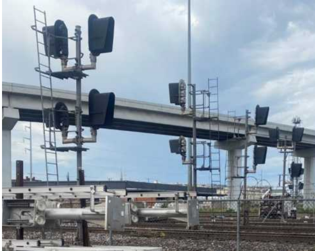
A row of signals span the North/South Bound Tracks at Tower 55.
