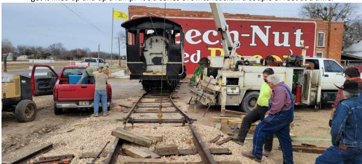
Above: The next step was to cut some rail and start blocking up. It’s almost on the permanent rail.
