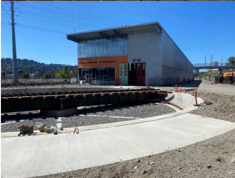
The recently installed turntable at the Oregon Rail Heritage Center (ORHC) was photographed in July 2023 and was awaiting installation of the motors to operate the turntable. Multiple tracks will be added as well. Photograph by Wayne Smith
