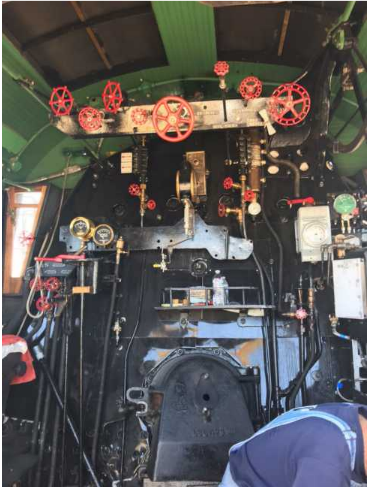
Inside the cab of 2926 - A worker is seen installing a more modern braking system. Also, see next page.
